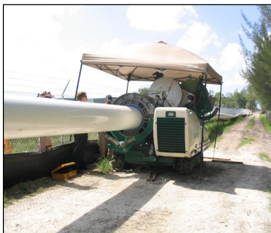
3,260LF 20” FPVC® Layout Adjacent to Airport
